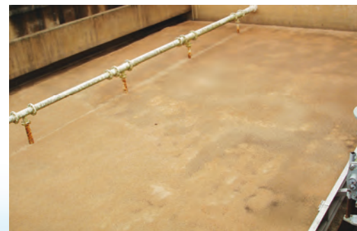
Figure 2.10 Sand filter in a water purification plant
